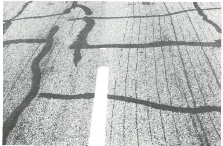
Job 2637 Shows Crack Pattern
