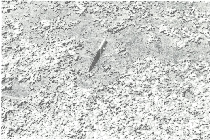
Job 2631 Shows Scaling after Resealing
