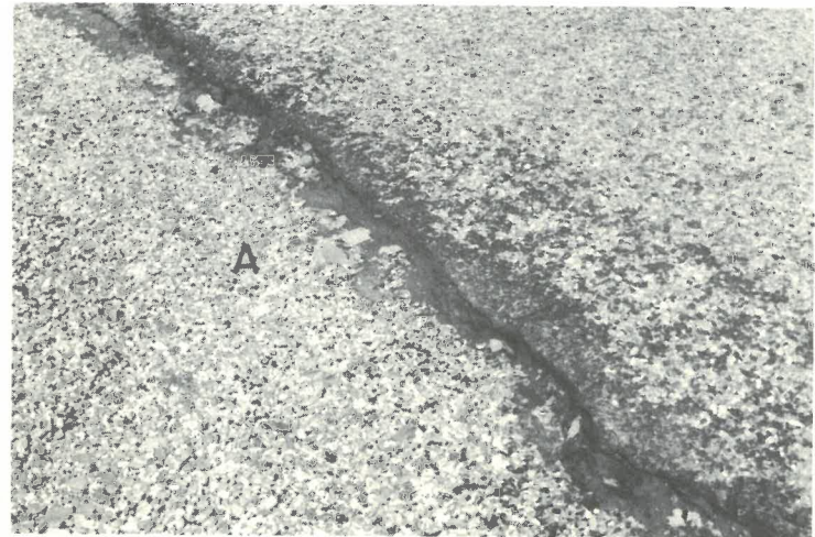
Job 7586 Shows a Change in Texture with Cracking
