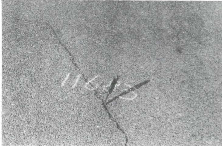
Job 11683 Longitudinal Crack Center of Lane
