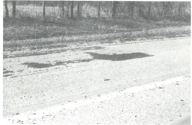
Job 2631 Shows Scaling after Resealing
