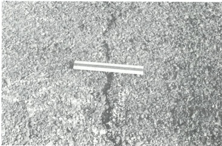
Job 2631 Transverse Crack
