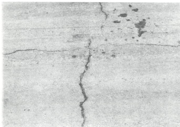
Job 11683 Longitudinal & Transverse Cracks
