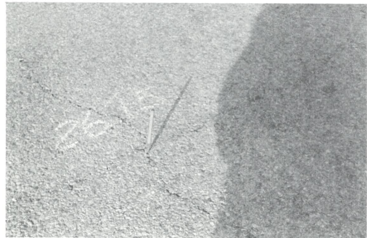
Job 2615 Longitudinal Crack
