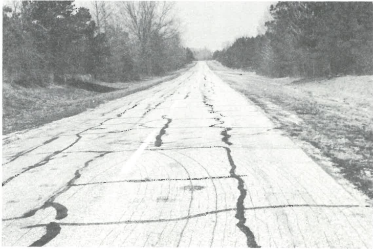
Job 2637 Shows Crack Pattern
