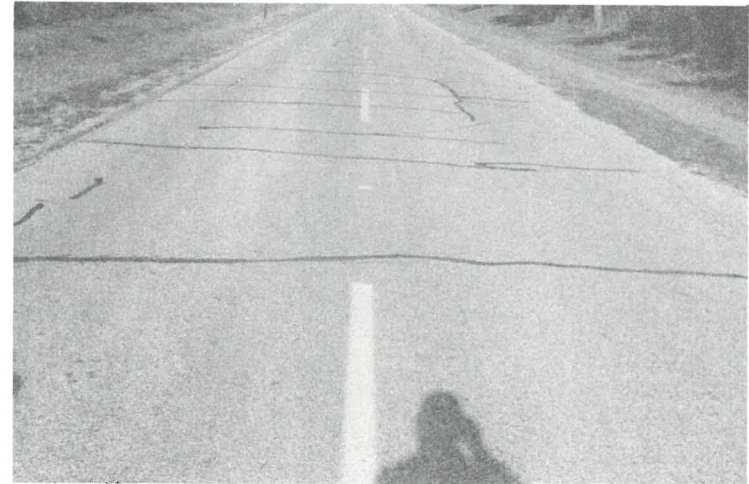
Job 2631 Transverse Crack Pattern of 6' to 12'
