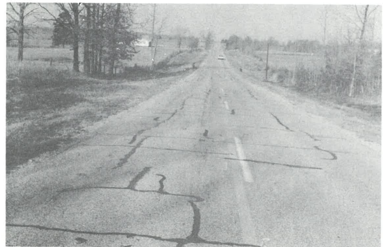
Job 2631 Logitudinal and Transverse Cracks
