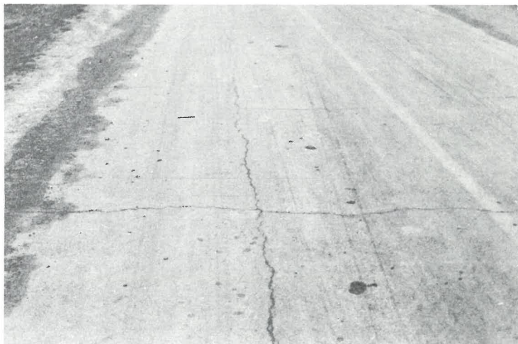
Job 11683 Longitudinal & Transverse Cracks
